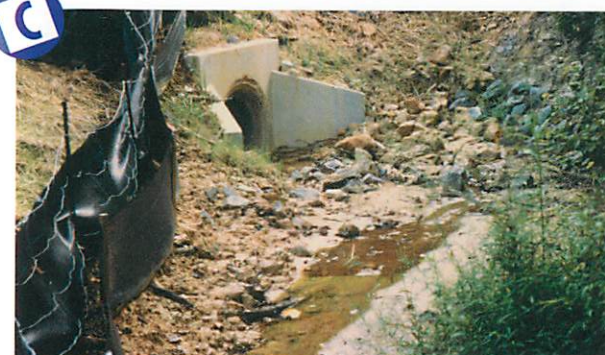
Poor geometry. Inadequate stone coverage.
