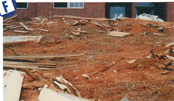
Completely inadequate coverage.
