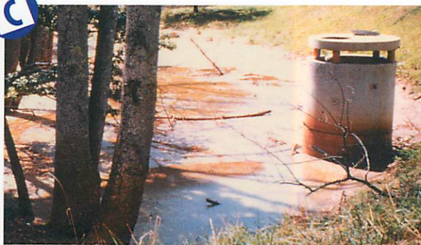
Poor outlet geometry. Potential maintenance problem.
