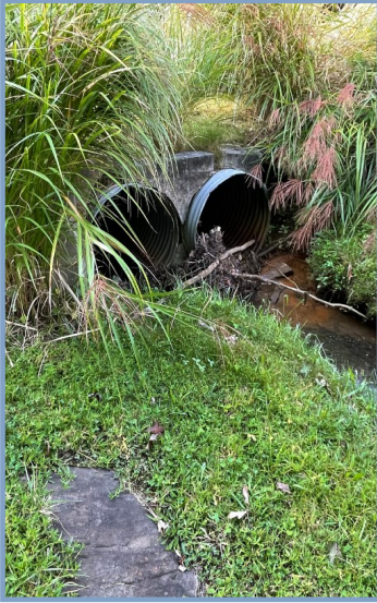
Pre-Construction: Twin corrugated metal pipes and head wall were failing.
