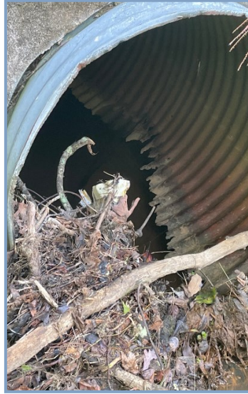
Pre-Construction: The bottom of both corrugated metal pipes had corroded away.
